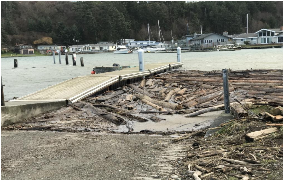
New pilings and unwanted logs
